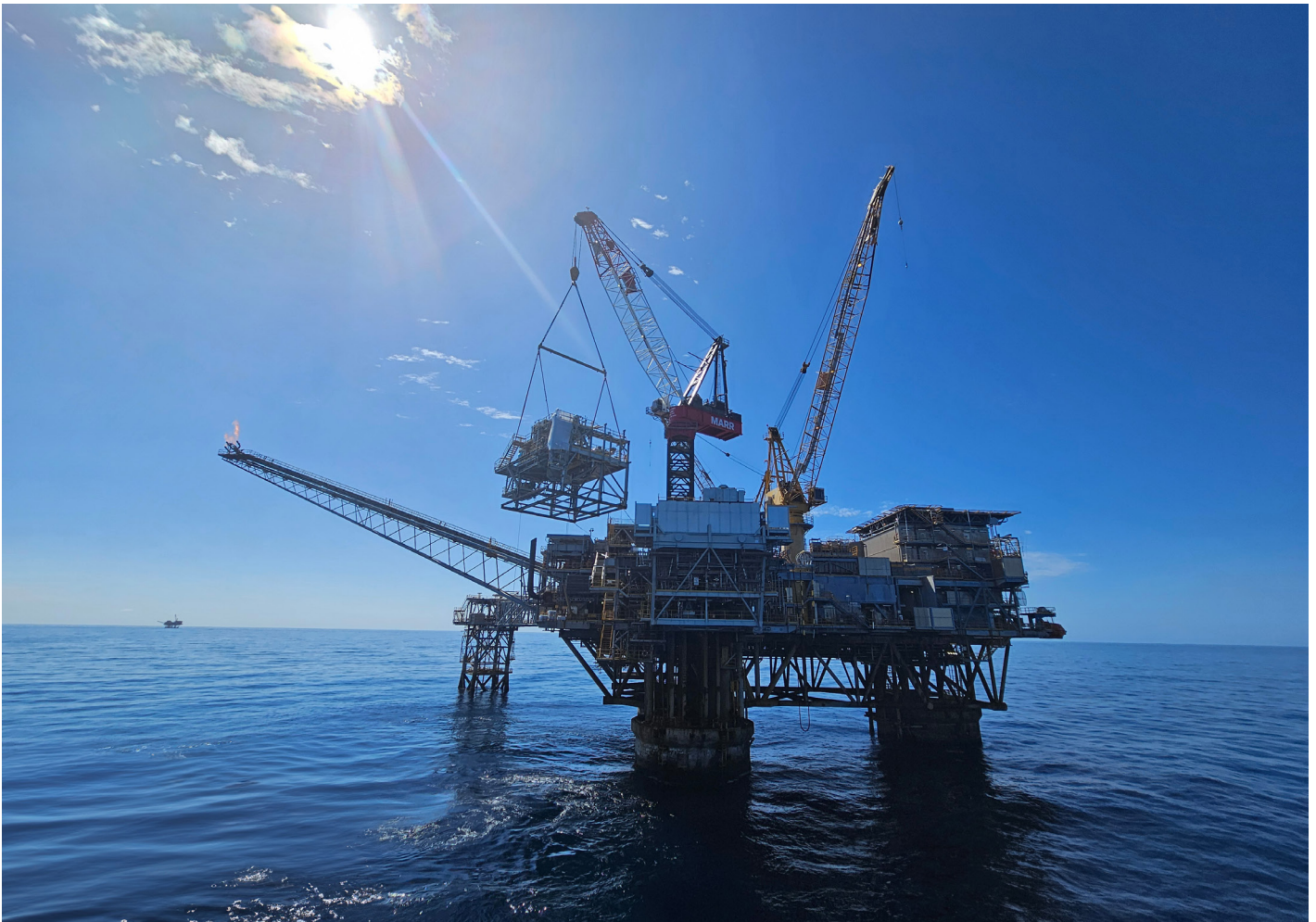
Marr's solution allowed heavy modules weighing up to 120 tonnes to be lifted from supply vessels onto the platform in varying sea conditions.
